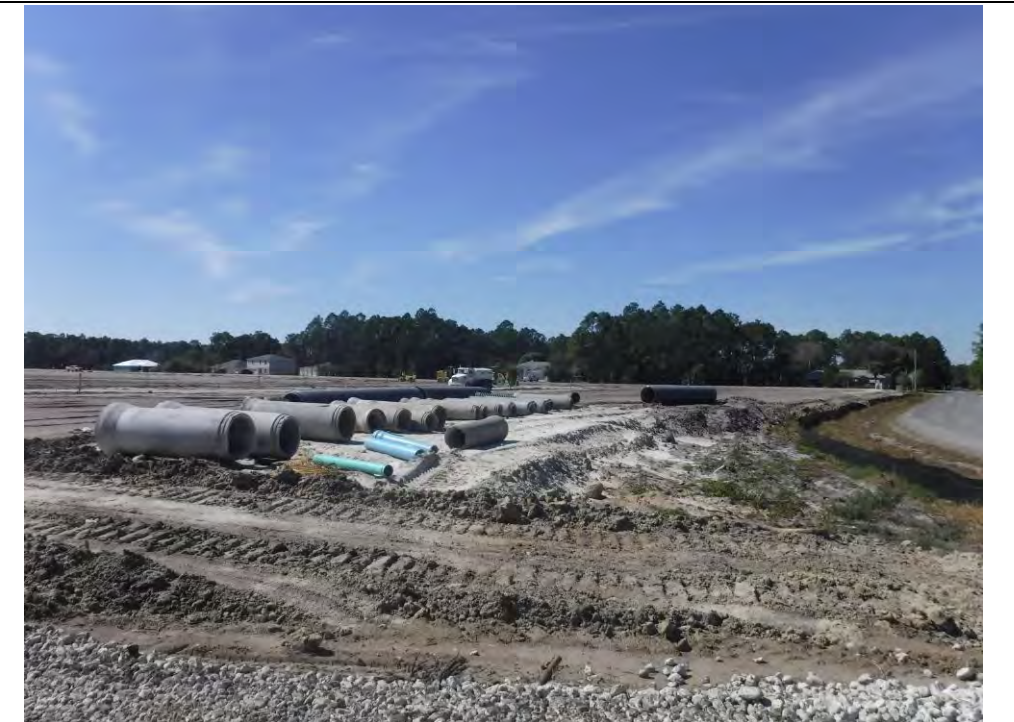
Photo taken from north of the site facing south. The area is under construction and currently contains concrete and PVC pipes.
